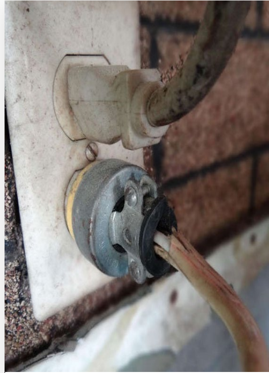
Figure 11-5: Damaged Electrical Cord
